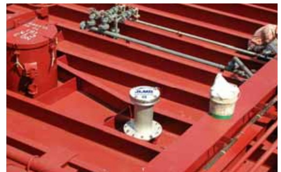
Photos from one of the ships that the JLMD System has been just installed - Sep 2004 Newbuilding launching - S.Korea
